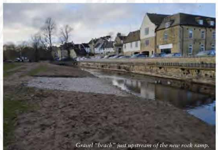
Work in progress: coir roll being installed to form a berm by the new rock ramp.
